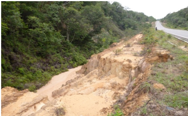
Figura 08: Voçoroca 13, km 43,5, BR174.
